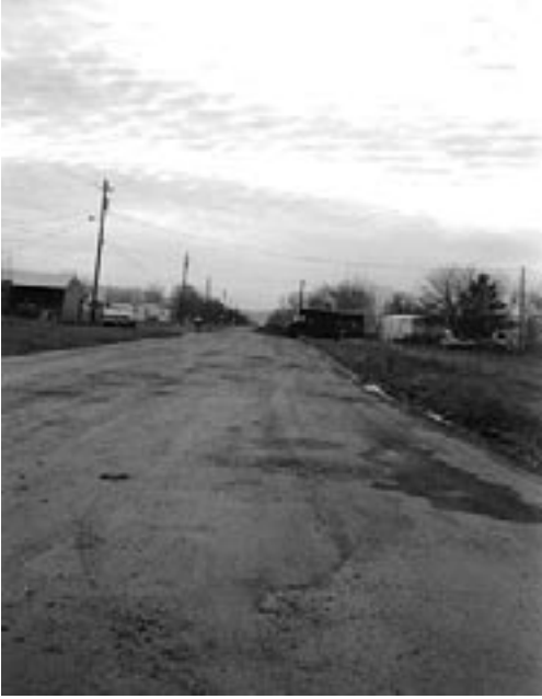
Avenue A in White City. The potholes here are not as bad as some areas. The street has been torn up and is being repaved.
